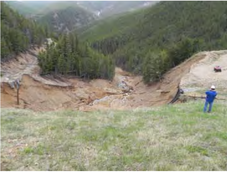
Alder Gulch Waste Dump failure looking downhill
